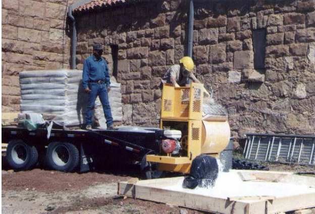
Ernest Martinez and Pete Mold mix high calcium hydrated lime into lime putty.
